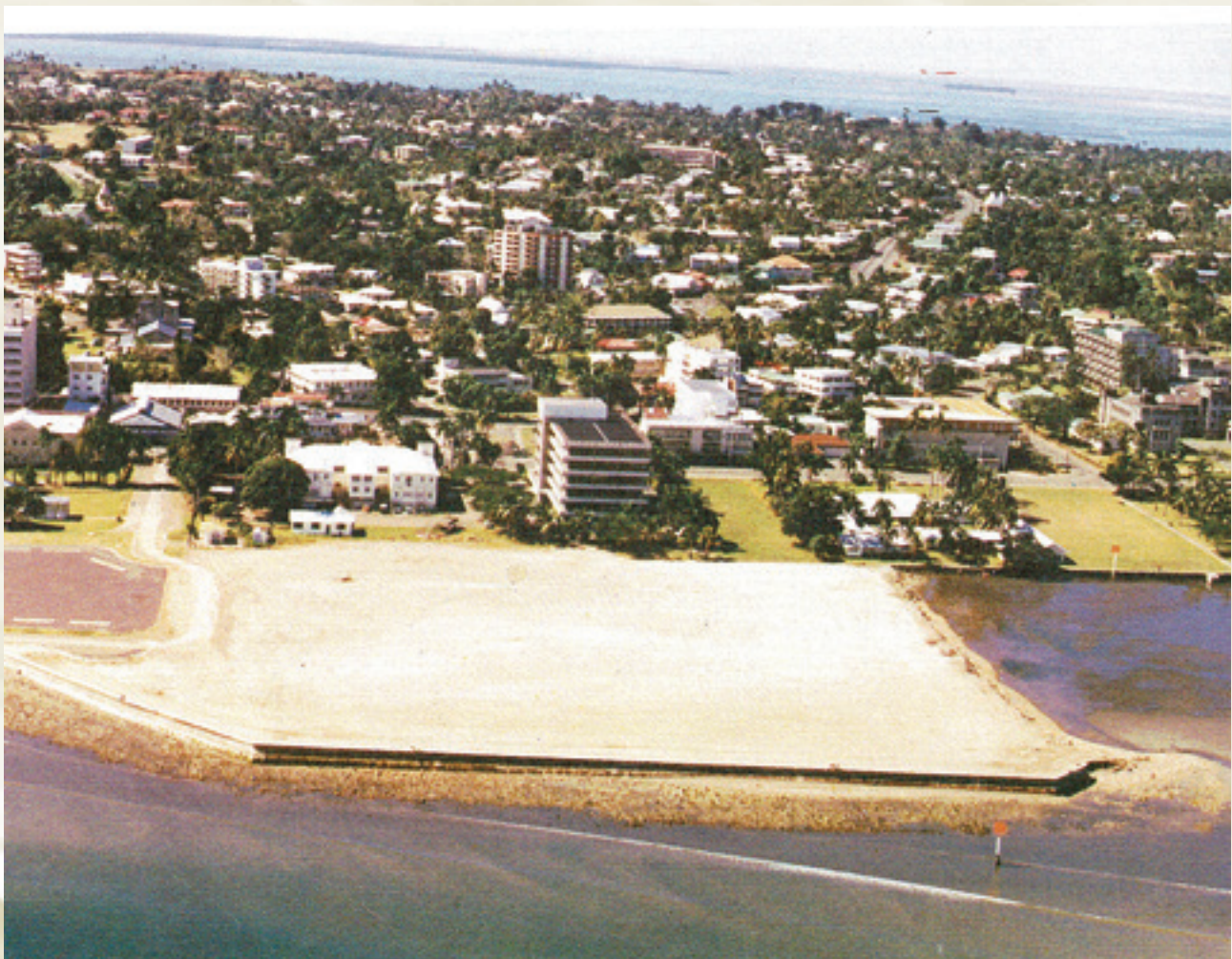
Reclaimed foreshore for the Hotel Development, in front of the Development Bank Centre.
