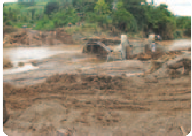
Remnants of the Moto Bridge in Ba after the January flood.
